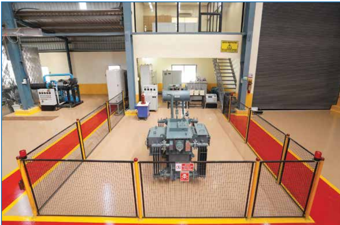
Testing Area with Transformer
